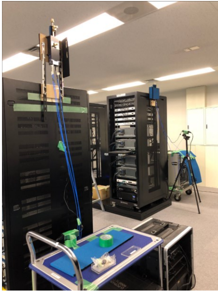
Data center measurement photo
