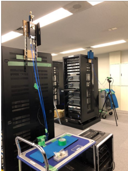
Data center measurement photo
