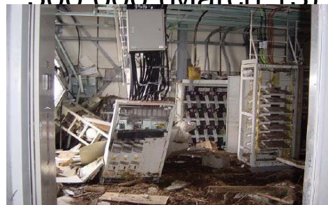
NTT DOCOMO transmission facilities in Iwate (Source NTT DOCOMO)
