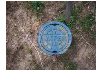
Typical Curb Valve Cover
