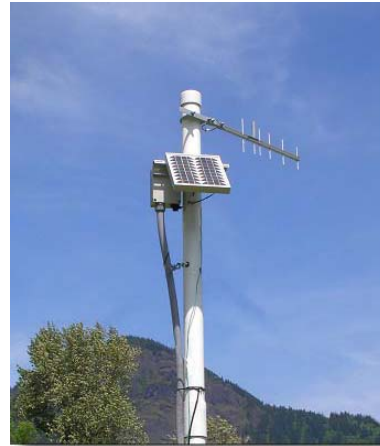
Data Collectors 20-30 ft above grade Placed 1-2 miles apart
